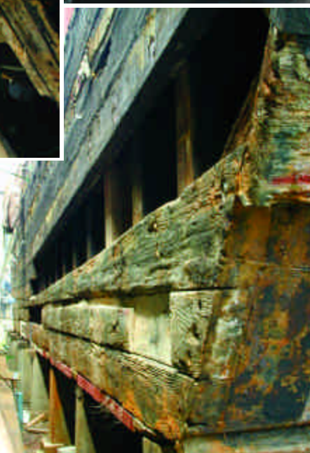
Worms, time and saltwater took a toll on the 87 year old barge. With restoration nearly complete, it has found new life as a waterfront museum, classroom, art exhibition center and reception hall. Photos © 2002 Frank Zimmerman and Doug Pierson
